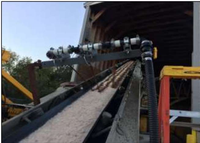
Figure 2: Stockpile treatment of salt as it is loaded in the salt dome.
